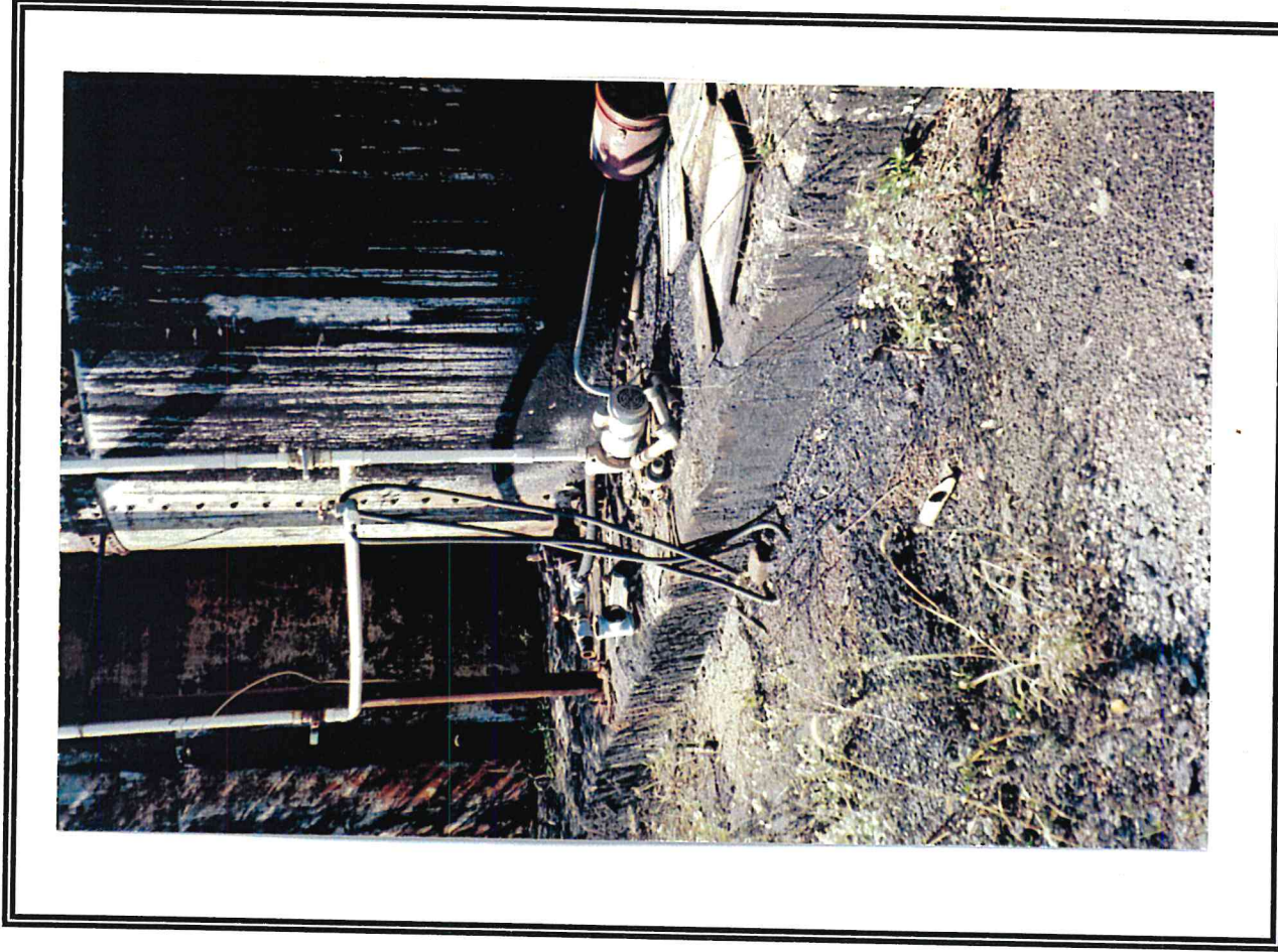
3. West AST area, facing southwest. Note stains on concrete pad and soil. Photo taken on 10/08/98.
