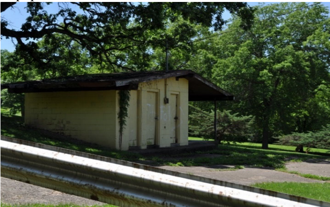
The current bathroom is beyond repair.
