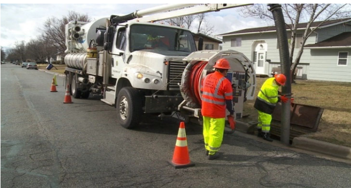
The vactor truck collects and transports sewage to the waste water treatment plant.
