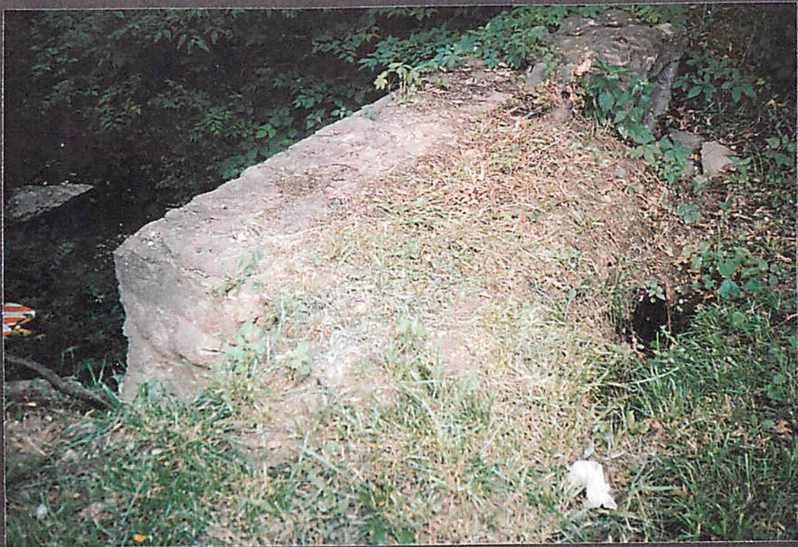
Looking at erosion around U/s face of stone arch culvert
