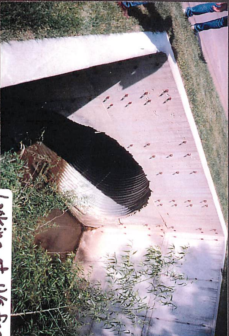
Looking ups at eroded toe on d/s face of culvert
