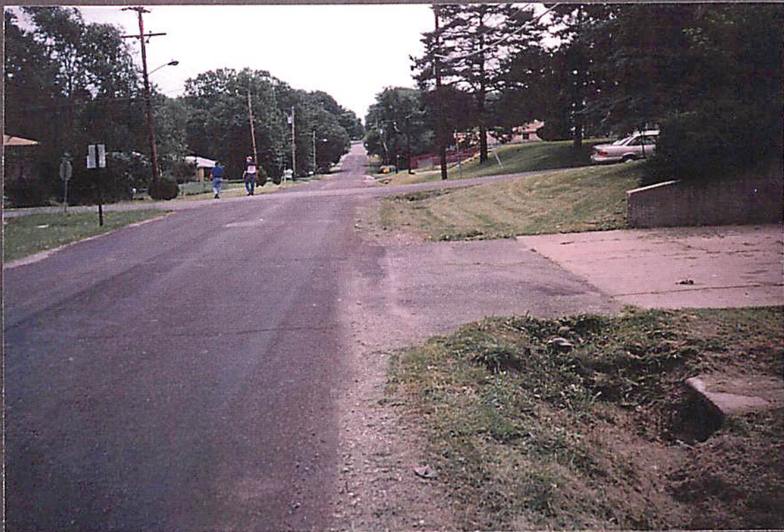
Looking east along Santa Fe St. west of Garland. Drainage tubes only on S. side
